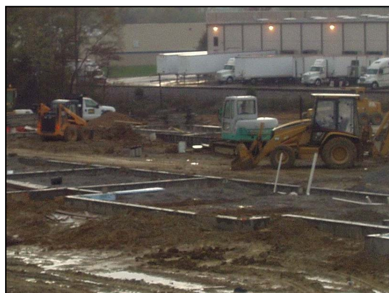
Despite rainy weather, construction continues on the residence halls. The halls are projected to be ready fall 2008.
